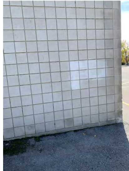
Photo 44 - East Elevation Block Wall Efflorescence
