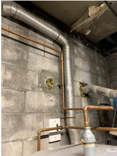
Photo 23 - Masonry Block Wall Efflorescence
