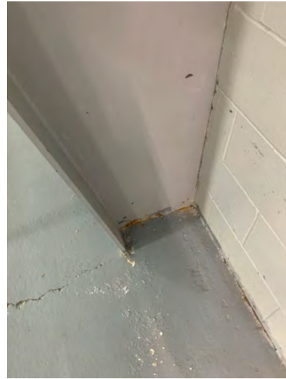
Photo 10 - Pre Engineered Frame Base Corrosion
