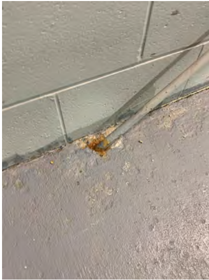
Photo 13 - Pre Engineered Frame Bracing Corrosion
