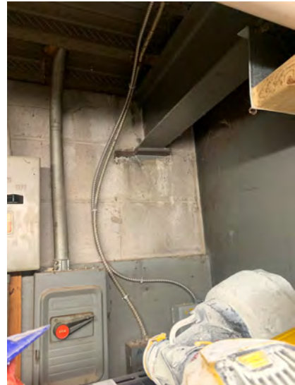
Photo 24 - Masonry Block Wall Efflorescence
