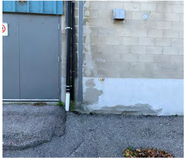
Photo 38 - South Elevation Block Wall Vegetation
