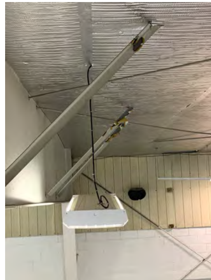
Photo 12 - Pre Engineered Frame Bridging Peeling
