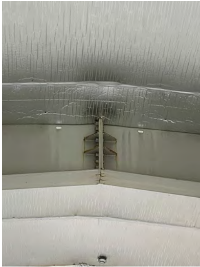
Photo 09 - Pre Engineered Frame Moisture Staining
