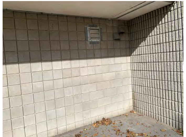
Photo 56 - West Elevation Block Wall Efflorescence
