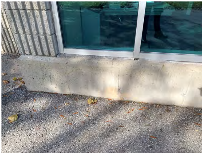
Photo 55 - West Elevation Foundation Wall Vegetation and Efflorescence
