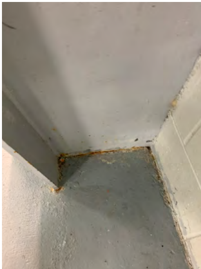
Photo 11 - Pre Engineered Frame Base Corrosion
