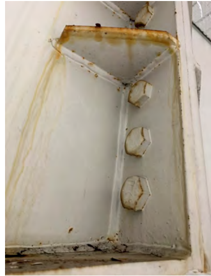
Photo 06 - Pre Engineered Frame Bolted Connection Corrosion
