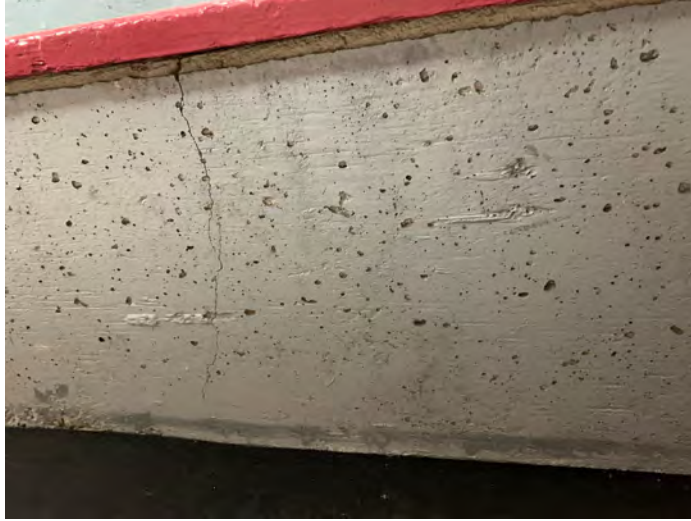
Photo 17 - Bleacher Seating Minor Cracking
