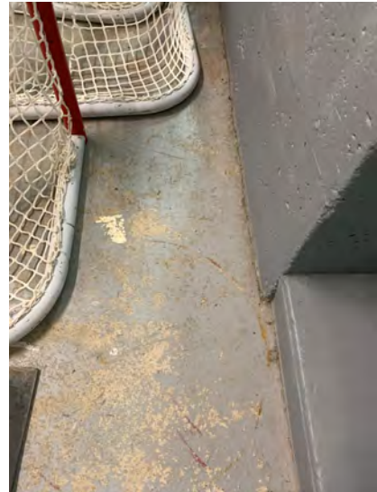
Photo 32 - Concrete Apron Slab Deterioration
