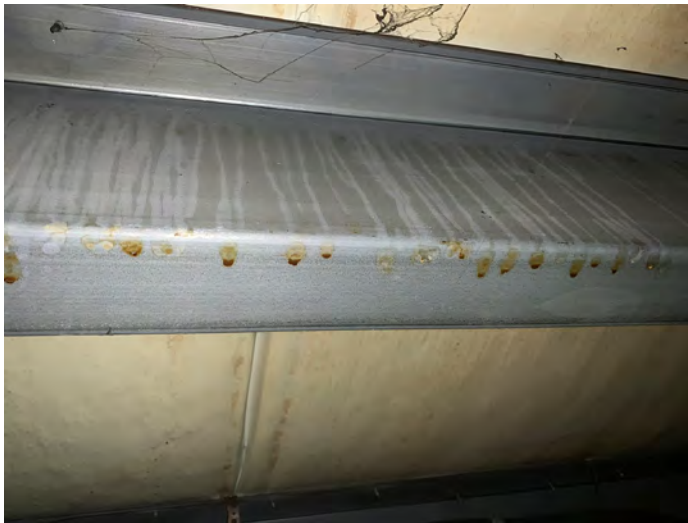
Photo 35 - Partial Second Floor Z Girt Water Staining
