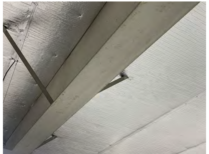
Photo 04 - Pre Engineered Frame Bottom Flange Corrosion
