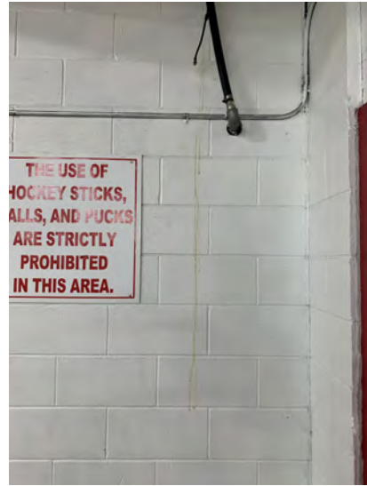
Photo 26 - Masonry Block Wall Staining
