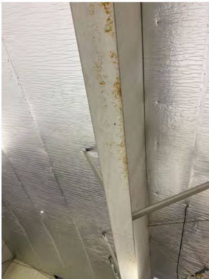
Photo 03 - Pre Engineered Frame Bottom Flange Corrosion
